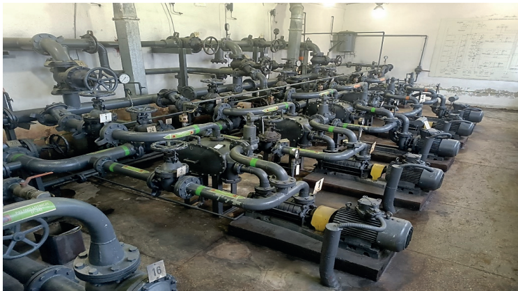
Fig. 5. Pumping units for fuel manipulation at the air base fuel depot
